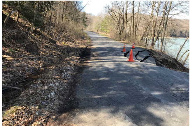
Hill slip along Beach Road.
