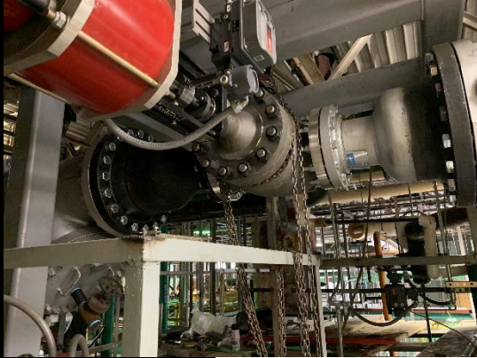
Ex. 2 ECSP As-Built Photo of Designed Condition
